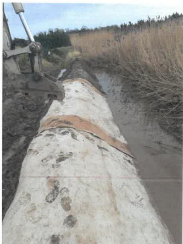
Picture 2 – Placement of new Geosynthetic Clay Liner (GCL) on the raised bund.
