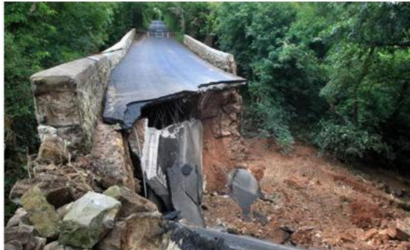
Bridge on the Iniscarn Road near Draperstown partially collapsed
