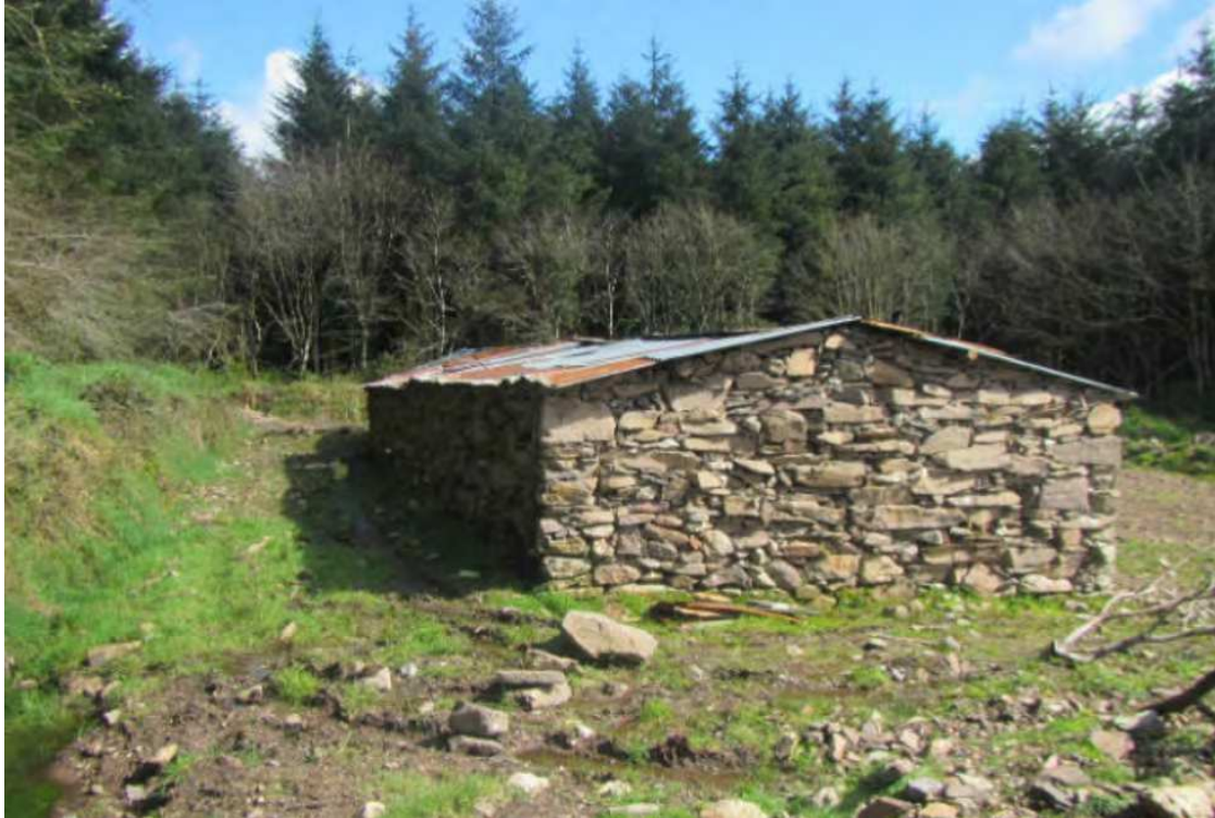
Fig 4: Photo of gable (southwest facing) elevation of the building to be replaced
