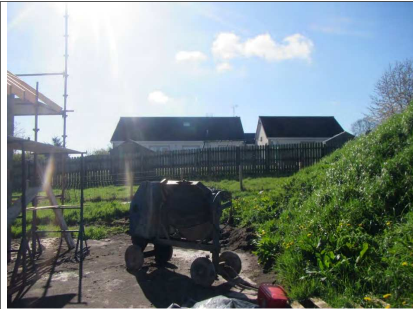
Figure 6 - View standing at the front of the dwelling and facing the rear amenity space of No.21
